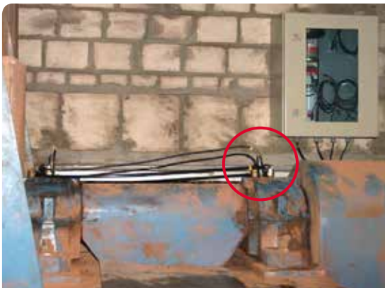
Lubrication system: perma PRO MP-6 (4 outlets activated)
