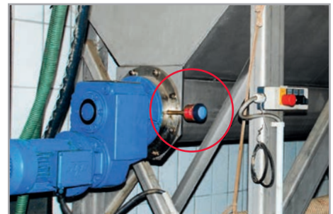
Sludge thickening process: Lubrication of bearing at screw press
